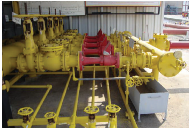
Fire Fighting System
