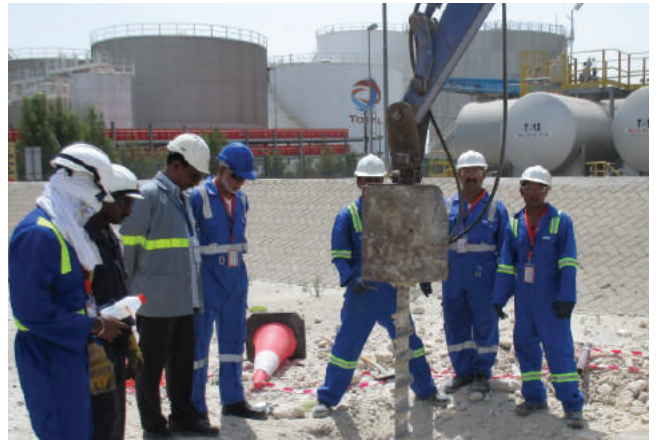
Ground Water Monitoring System
