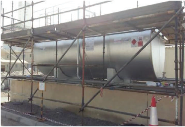
Flow Meter Installation
