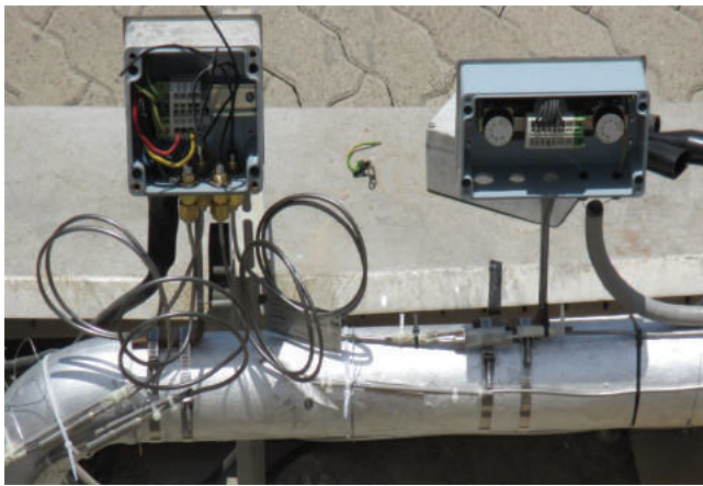
Electrical Heat Tracing System
